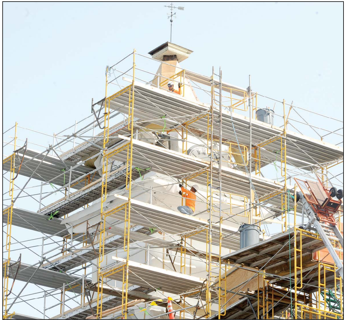
Workers with Renaissance Roofing continue their effort to restore the Edwards County Courthouse Clocktower Monday afternoon. Photo by T.J. Hug.
